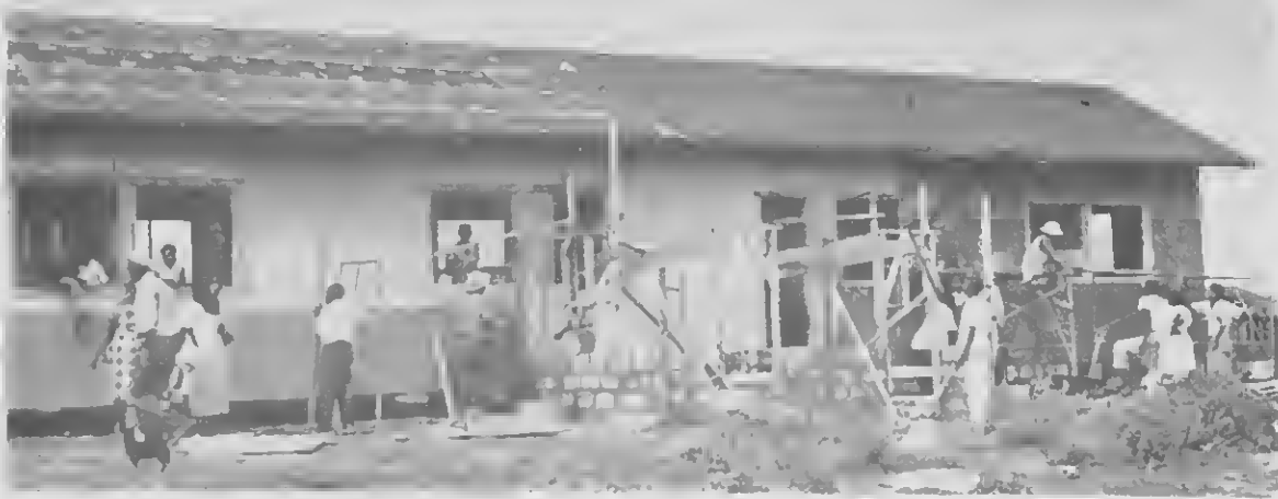
EVERYONE WAS busy during the work. This picture shows the entire building.
